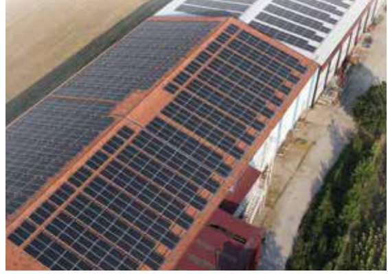
ERCAN MANAV 410KWp ÇATI - DENİZLİ
